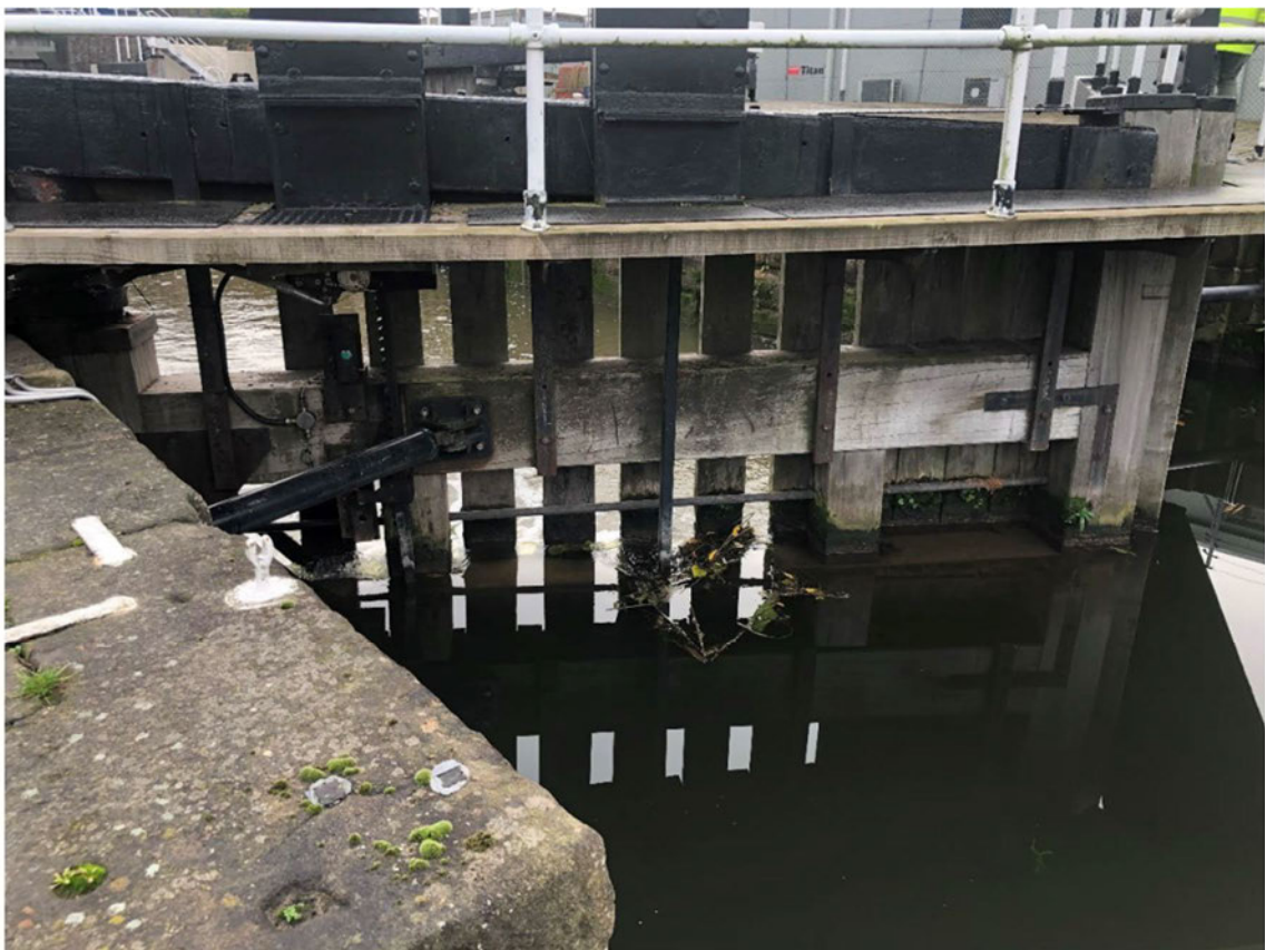
Figure 4 - Upstream face of the top lock gates to be modified at Keadby Lock (image Arcadis 2022)
